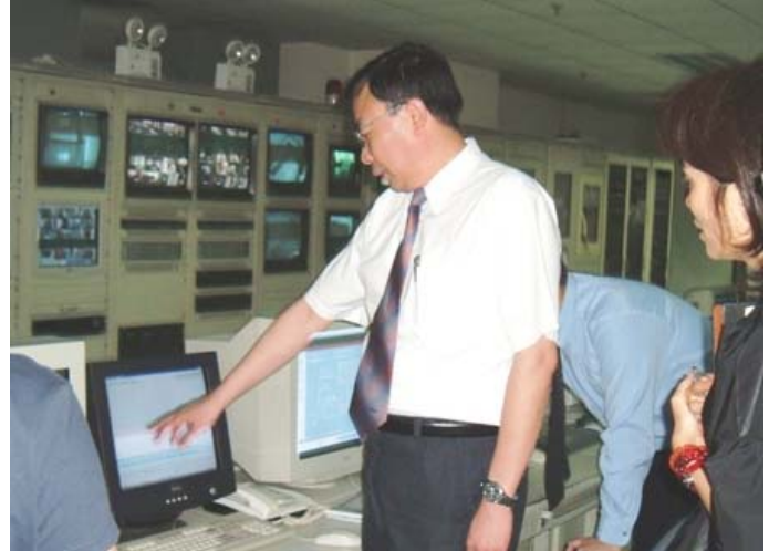
A Shanghai building manager discusses his commercial building’s automation system and energy consumption during a walk-through assessment.
