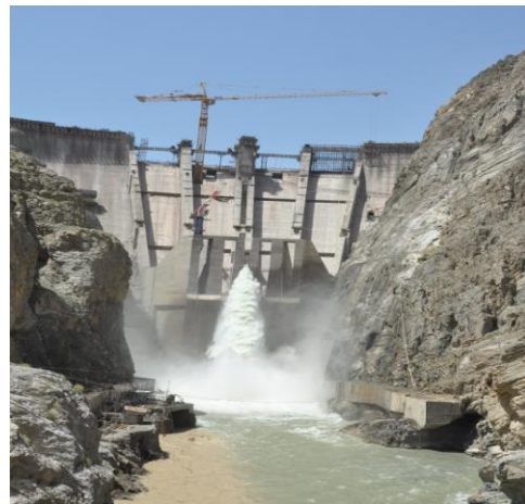
Gomal Zam Dam in South Waziristan is being built with support from USAID
