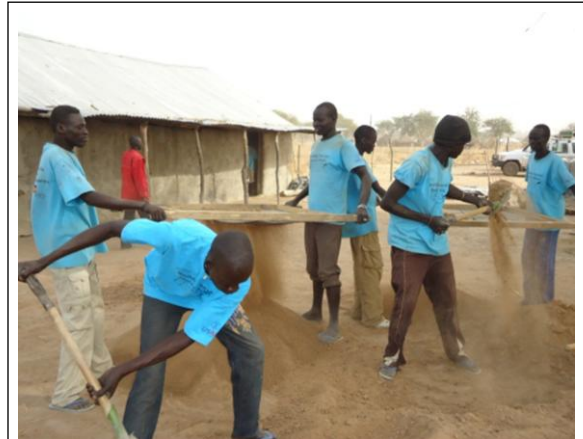
USAID supported youth from cattle camps in Panyijar County, Unity State, who produced high-quality compressed soil blocks for the county headquarters office—giving the youth a productive alternative to cattle raiding and providing infrastructure and visibility for local authorities who can help prevent conflict.
